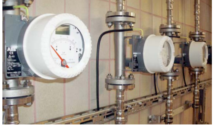
Variable area measurement of oxidation air in a water plant
