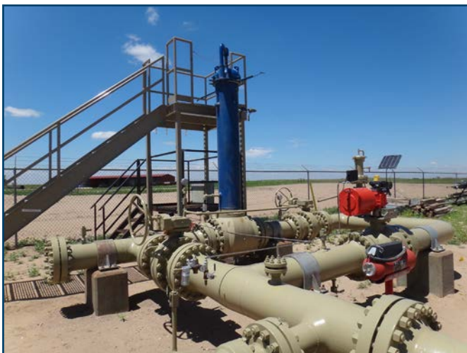
Colorado, USA 12 inch 600 ASME, five pig capacity Pneumatically actuated
