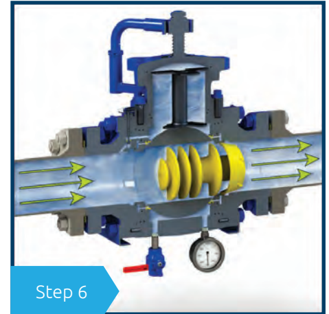
Step 6 Now in the open position, pipeline flow and pressure moves the pig downstream.
